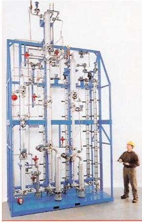
Still Mounted Continuous Purification System with 3" and 4" fractionating columns, plus absorbers, dessicator columns and control elements.
